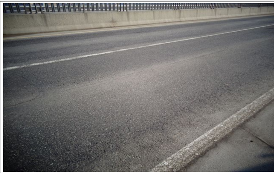
S11 망상균열 (원주방향)
